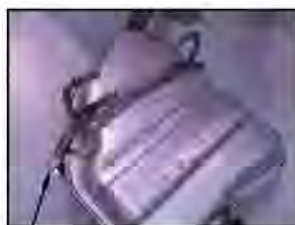
HANGER STRAP (TO BE REMOVED)
